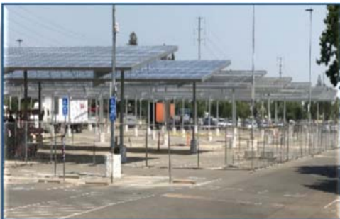
Solar Photovoltaic System Project: Yuba College
